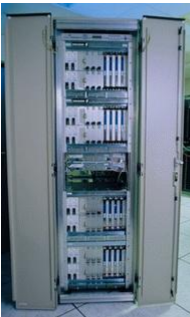
Figure 2. Telecom-Grade HW Used to Test JFS on Linux
