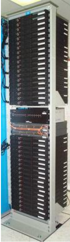
Figure 1. 1U Rackmount Units Used to Test JFS
